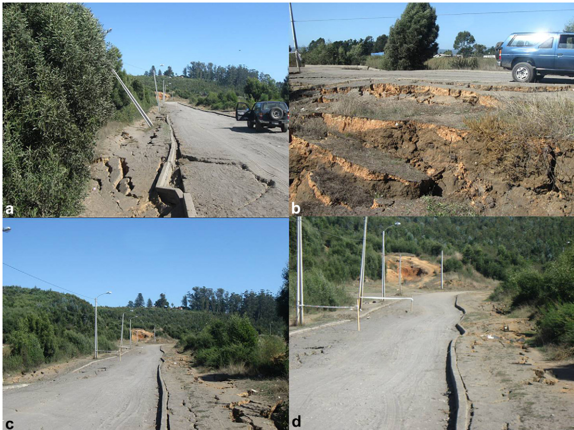
Fig. 2. Deformed ground due to Love waves in the city of Coronel ( 37^{\circ} S). The soil is soft and the orientation of the road is N10°E. a, b) Normal faults and open cracks. c, d) Undulated road, open cracks and normal faults.
