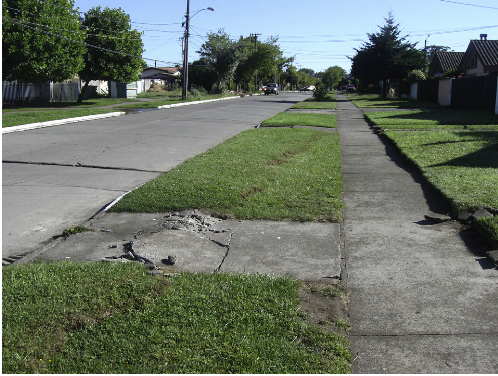
Fig. 1. Reverse fault scarp ( \sim N–S) generated during E–W movements due to Love waves and the different strength between the soft soil and the concrete of the roadway.
